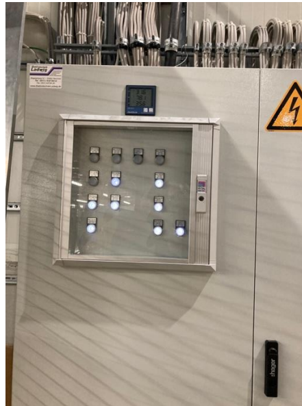
22- Central control of lighting
