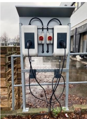
13- Wall box at the logistics site
