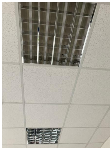
26- Canteen area lighting
