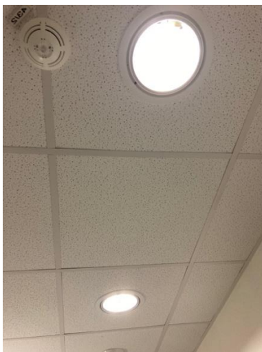
25- Lighting sanitary area
