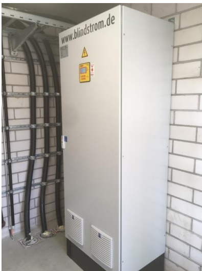
10 power factor correction system
